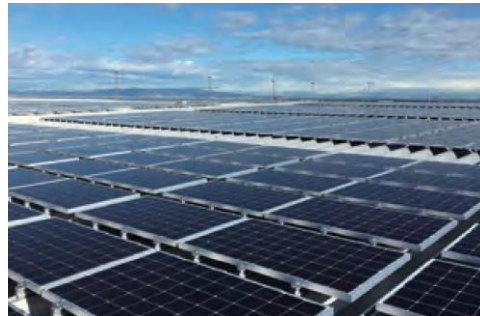
Introduction of solar power generation
