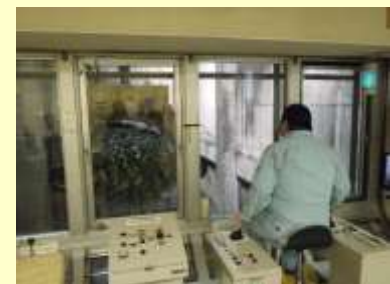
Central control room
