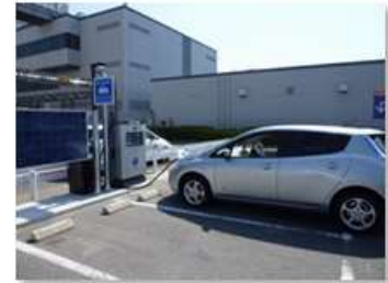
EV rapid charger, at Observation Hall
