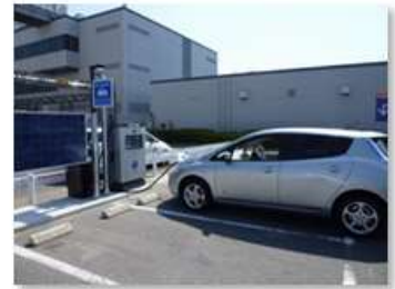
EV rapid charger, at Observation Hall
