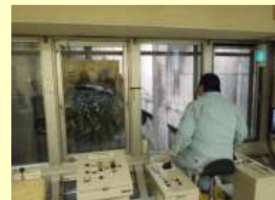
Central control room
