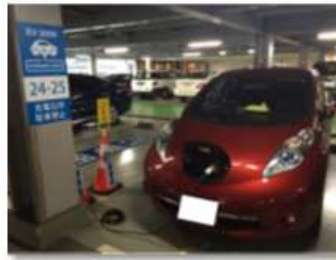
EV regular charger in parkade
