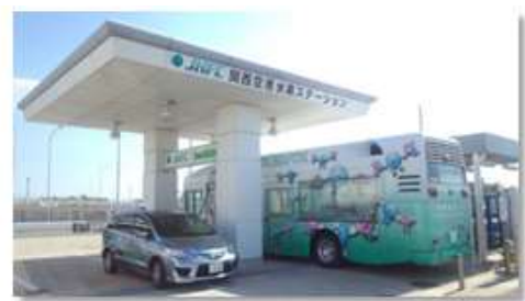
Hydrogen fueling station
