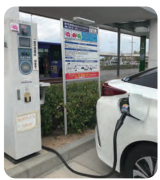
EV Charging Stations
