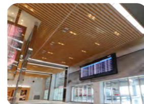
LED lighting in the terminal building (ITAMI)
