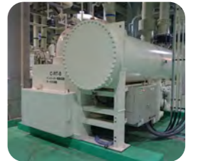
Inverter-controlled turbo chiller
