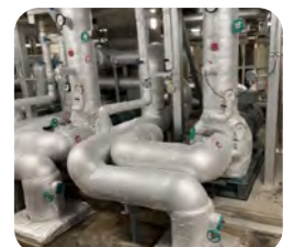
Cold- and hot-water pumps for air-conditioning
