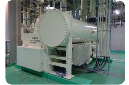
Improve efficiency of air-conditioning equipment
