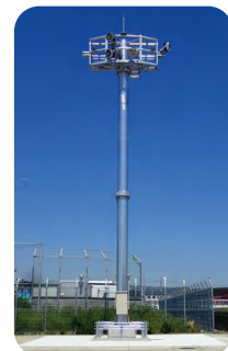
Apron LED lighting (ITAMI)
