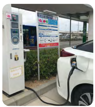
EV Charging Stations
