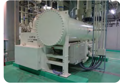
Improve efficiency of air-conditioning equipment
