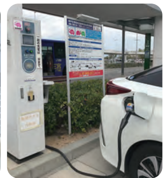
EV Charging Stations
