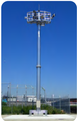
Apron LED lighting (ITAMI)
