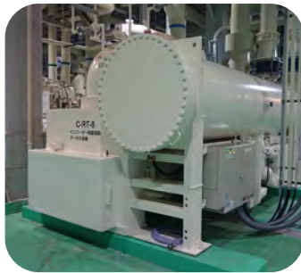
Heat-supply inverter-controlled turbo chiller
