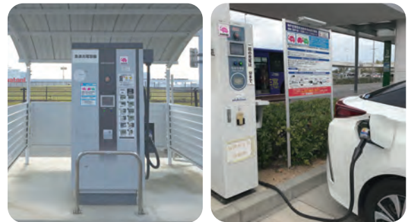
EV Charging Station
