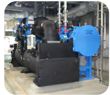
Inverter-controlled turbo chiller
