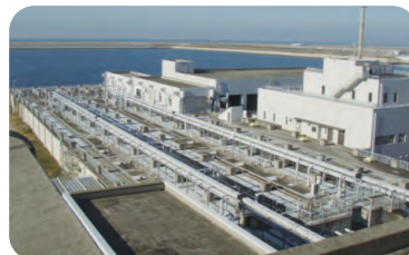
Sewage Treatment Center
